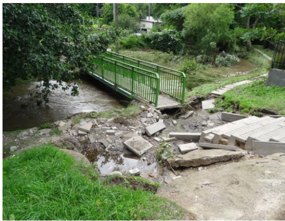
Figure 2.6. Destroyed entrance to the bridge on Kacza. Own photo
